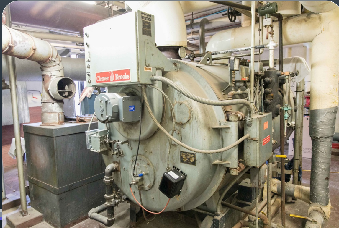
Lincoln Elementary, built in 1911; boiler beyond its useful life
